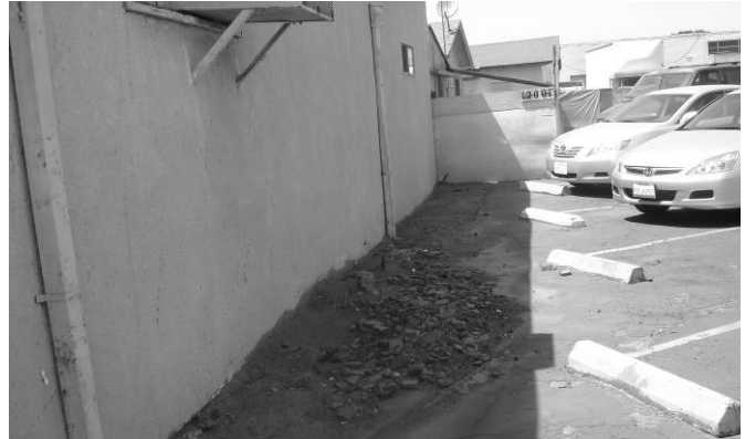
Deteriorating parking lots containing uneven surfaces
