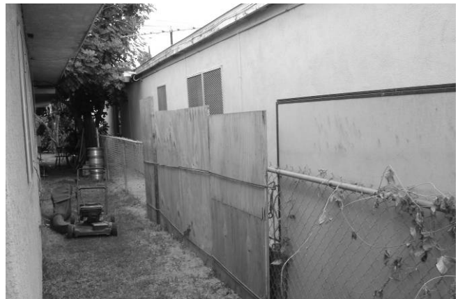
Prohibited fencing materials
