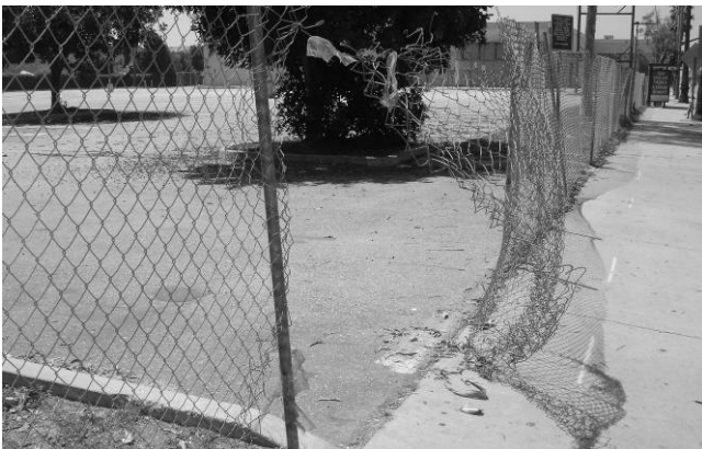
Fences which are in a hazardous condition
