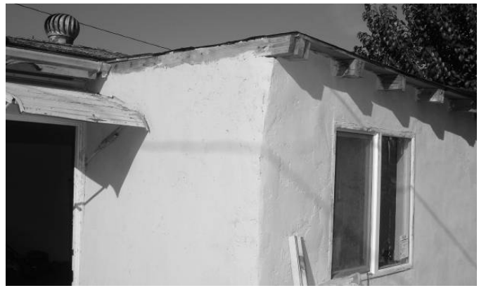
Illegal addition, no permit
