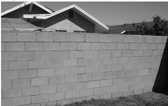
Illegal block wall, no permit
