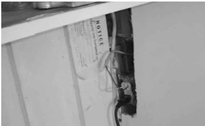
Illegal electrical work, no permit
