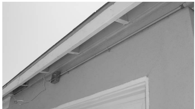
Illegal electrical work, no permit
