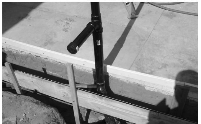
Illegal plumbing, no permits
