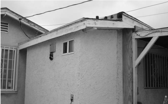
Illegal house addition, no permit
